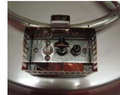
Top View- note next to burner
